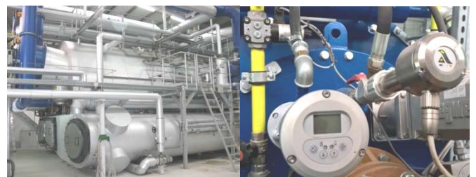
Fig.1 The boiler of the GETEC Heat & Power AG and sensors on the front part of the boiler.
